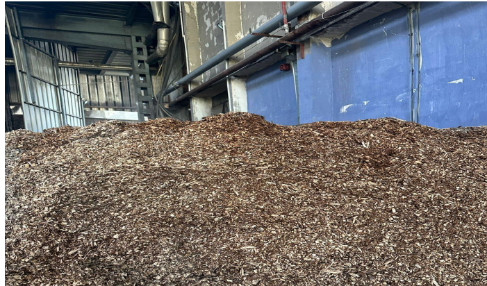
"BIOMASS: AGRO WASTE FUEL" fueling Nahar's boiler system (Rs 4.70/KG)
